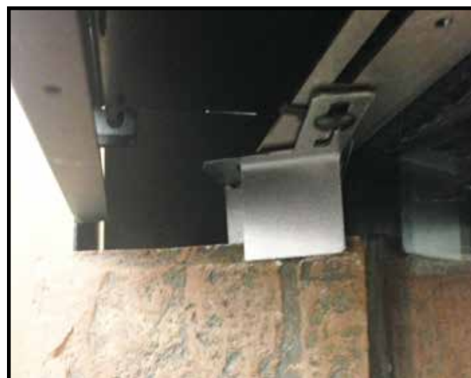
Figure 7. Side Refractory Brackets
